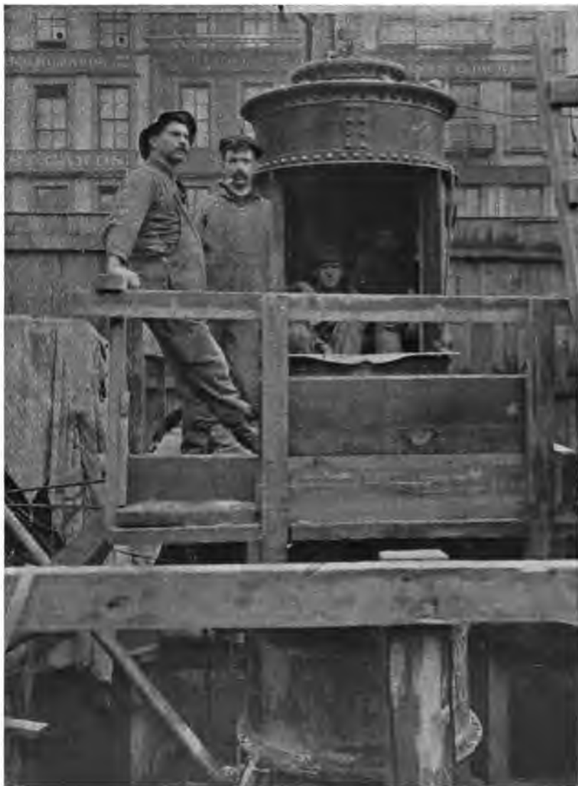
PLATE 230. —Contract 67. Shaft 19. Mattsen Air Lock in Position Over Shaft Leading to Working Chamber of Concrete Caisson. Lock is closed by a revolving door fitting opening and a trap door at bottom,
